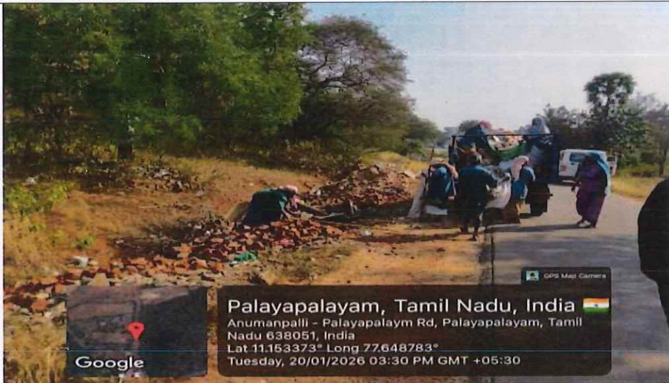
Cleaning and removal of the dumped waste was being carried out manually by Chennimalai, Block Development Officer
